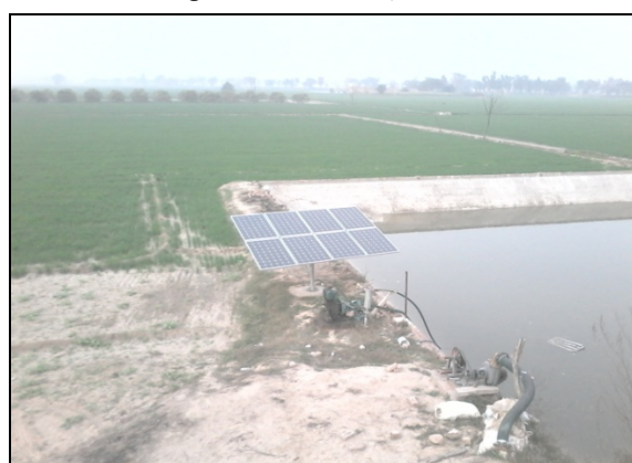
Fig. 4: Solar based drip irrigation system
